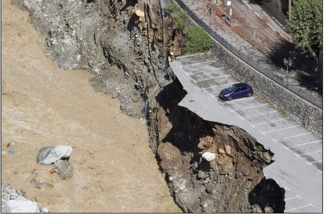
Şekil 43. Fransa-Saint-Martin-Vesubie'de Sel Hasarı (3 Ekim 2020) ( https://www.theatlantic.com/photo/2020/10/photos-flooding-southeastern-france/616629/ )
